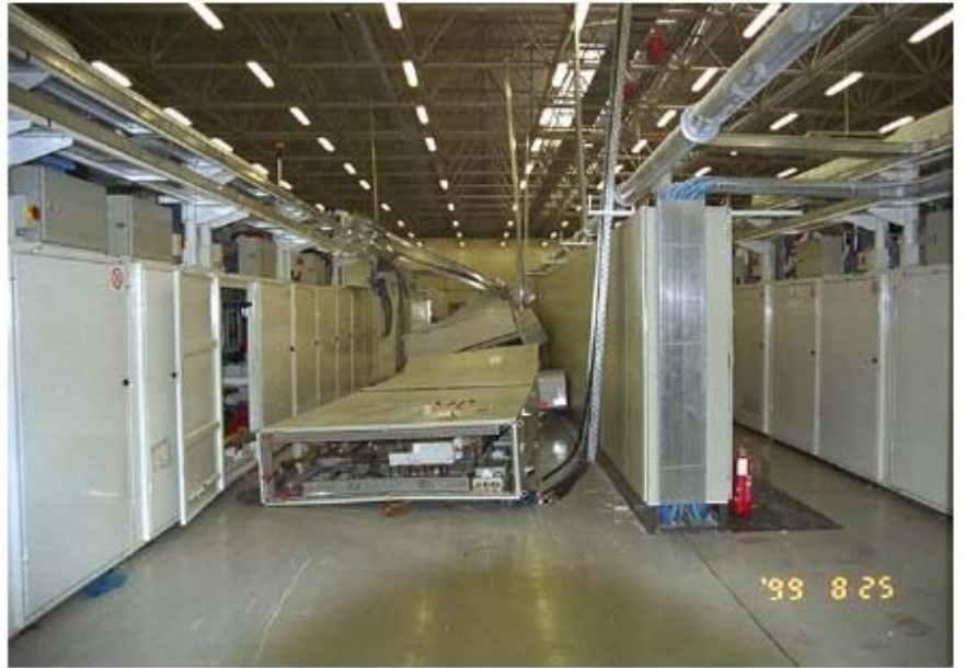
1999 Izmit Turkey, earthquake
