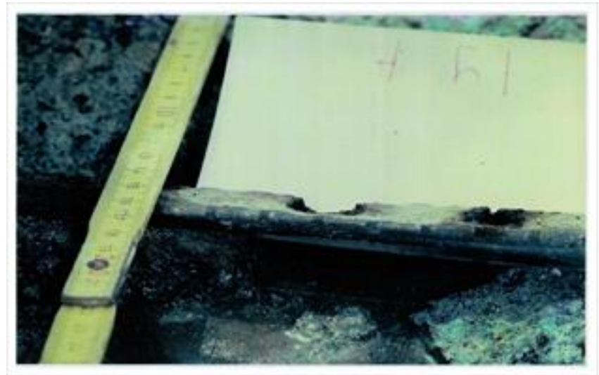
Typical corrosion attack in a bridge deck with high chloride concentration
