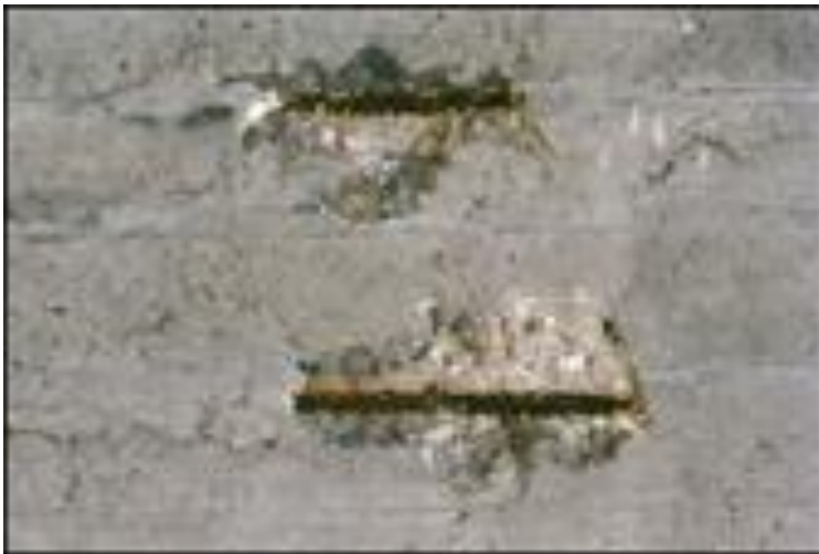
Uniform corrosion with rust formation
